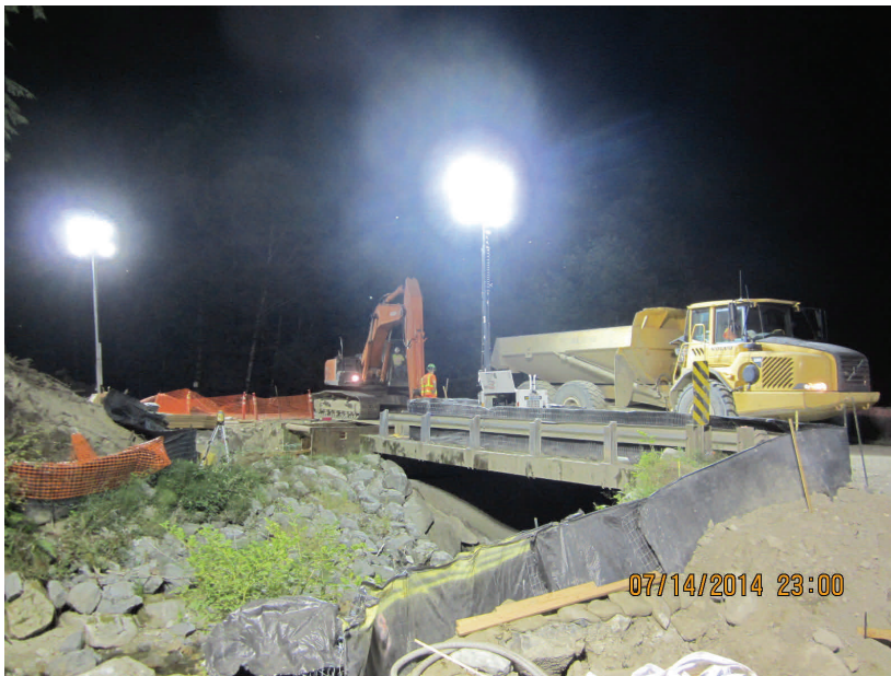
Above: Night shift preparing to divert the stream and remove the existing bridge at 588+50.
