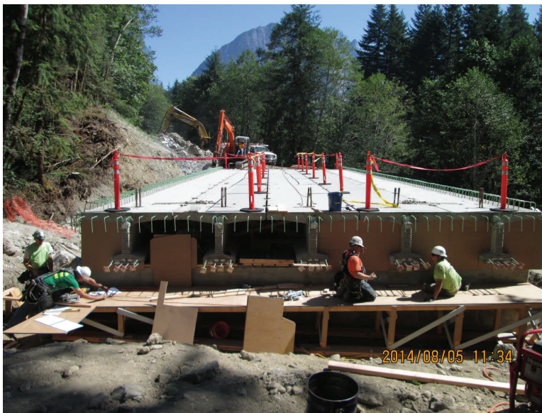
Above: Building concrete formwork at the 588+50 bridge and excavation in the background.
