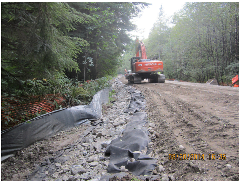
Above: Placing rip rap so the roadway can be widened over soft soils.
