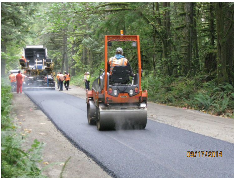
Above: Paving between the Middle Fork Trailhead parking lot and Middle Fork Campground.
