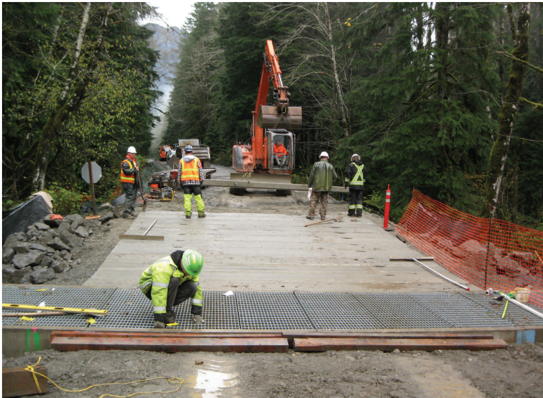
Above: Installing low water crossing planks. These armor the roadway so it will not wash out in extreme flood events.
