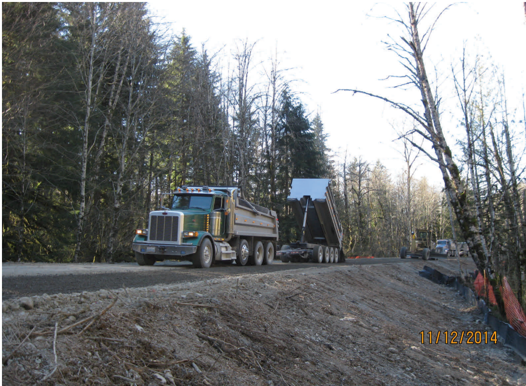
Above: Placing crushed rock on the completed roadway embankment near the beaver ponds.
