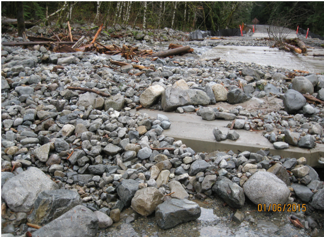
Above: Flood debris blocking roadway.
