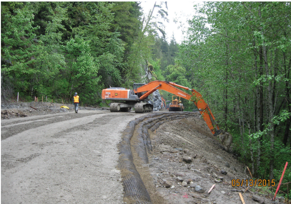
Above: Constructing a reinforced roadway over the slide near the CCC trail.
