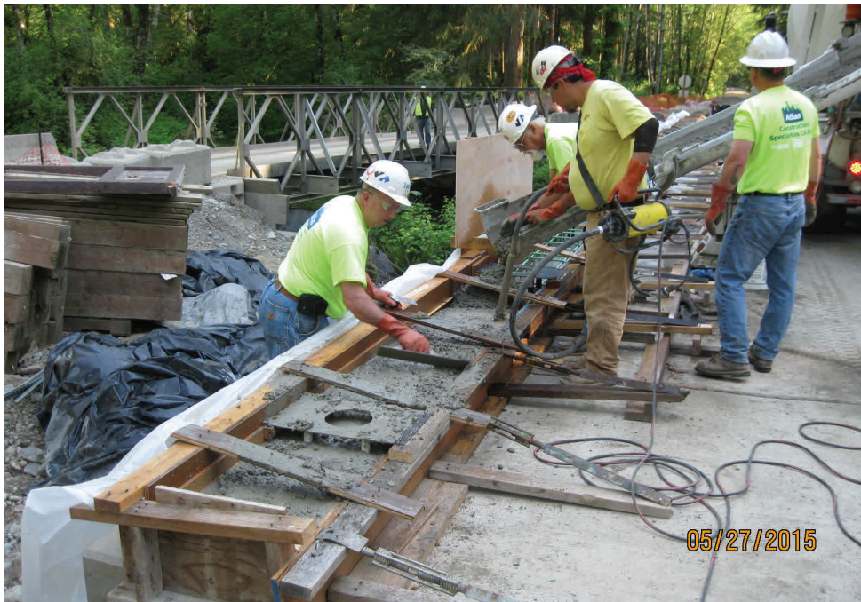
Above: Pouring concrete bridge rail curbs on the new Big Blowout Creek bridge.
