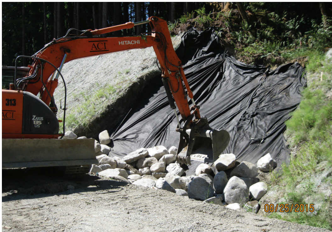
Above: Placing rock to stabilize a slope that slid during last winter's heavy rain.
