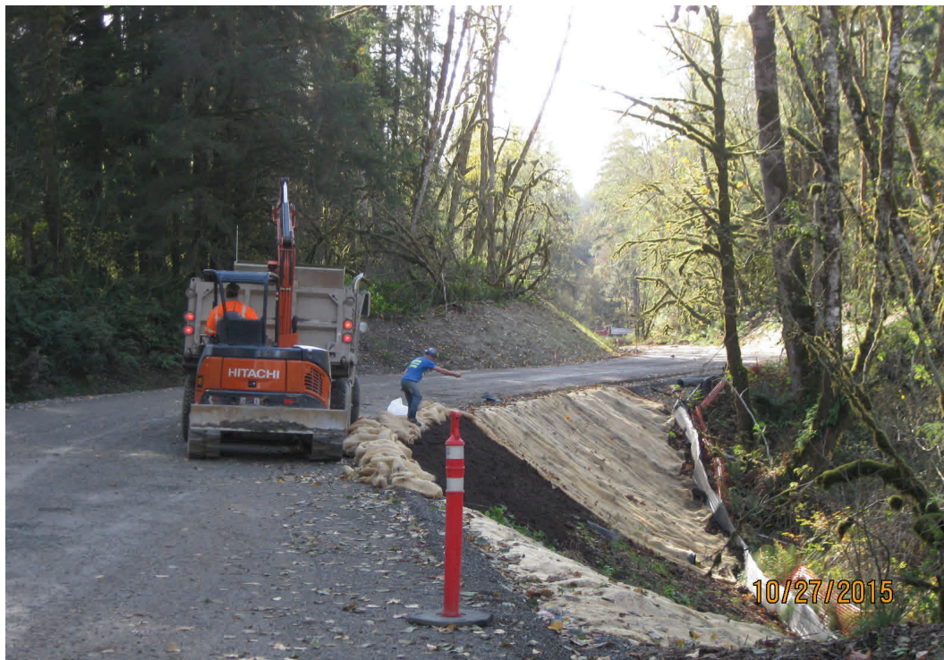
Above: Placing topsoil, seed, and erosion control fabric on a finished slope.
