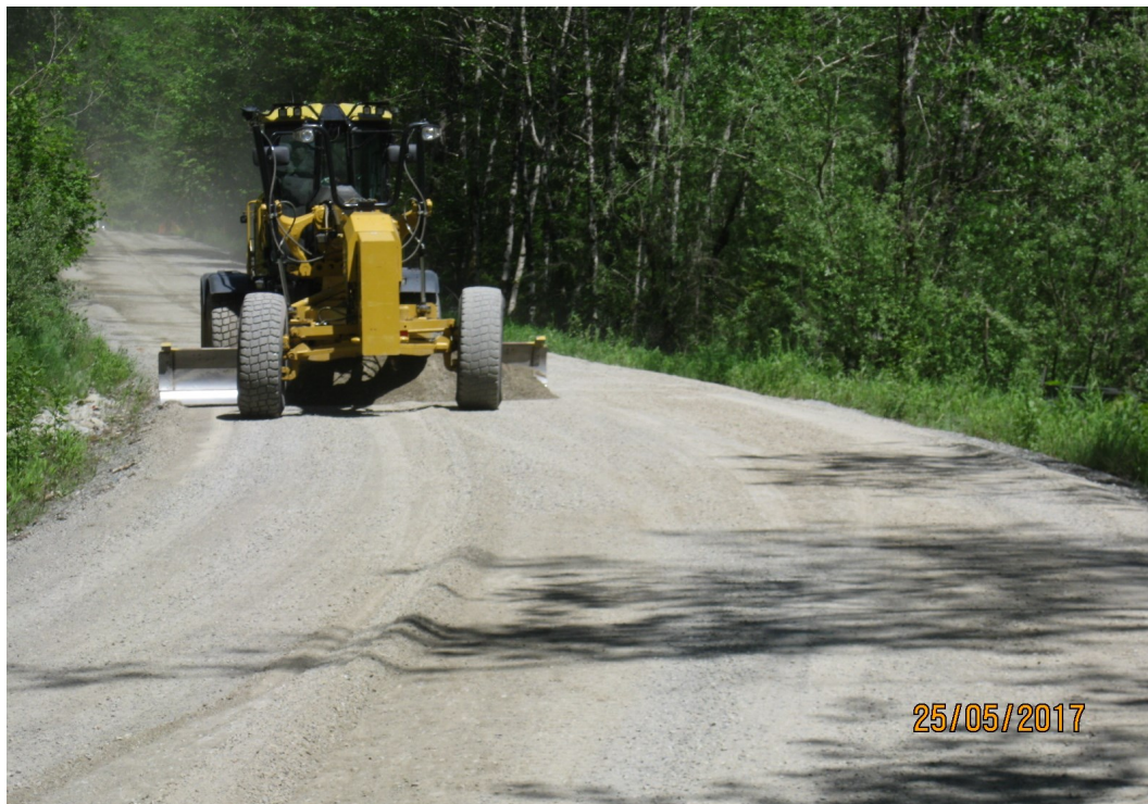
Above: Grading surfacing near the CCC trail to prepare for asphalt surface treatment.
