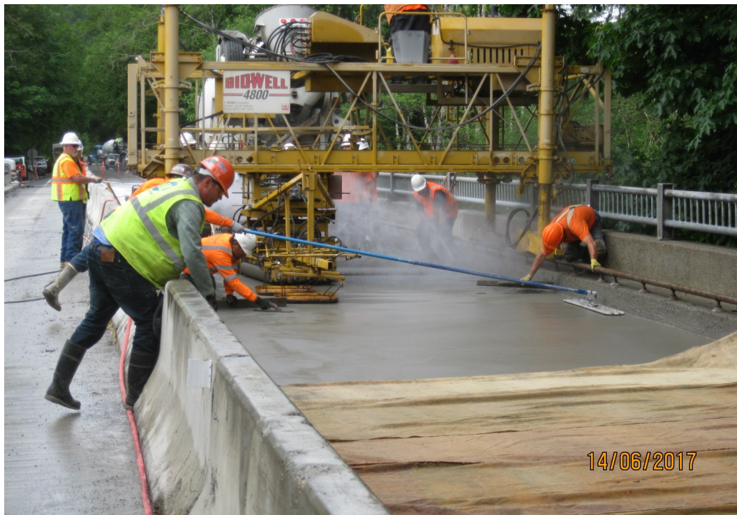
Above: Placing the second half of the Lake Dorothy bridge concrete deck overlay.
