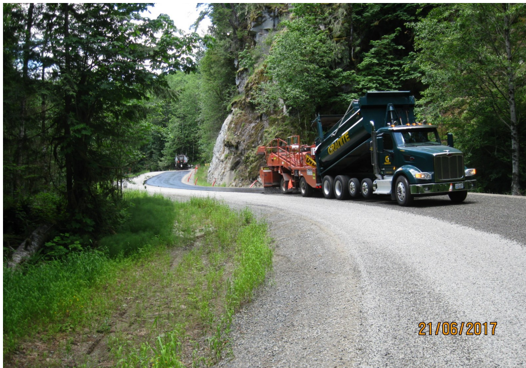
Above: Placing the first layer of asphalt surface treatment near the CCC trail.
